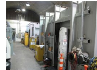
Indoor Battery Test Facility
